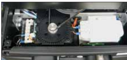
Fig. 2: Lamp ballast and voltage tapings
