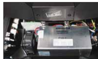
Fig. 19: Lamp power supply.
